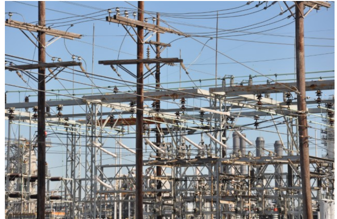
Electrical power substation (DHS)
